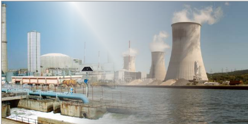
Use of ELN BAR In Water Intake Flow & Pressure Measurements in Nuclear Power Plant
